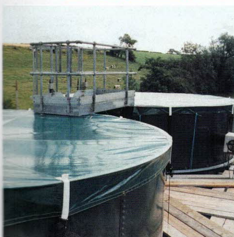
Sludge digestion tank covers at Severn Trent Water Authority site.
